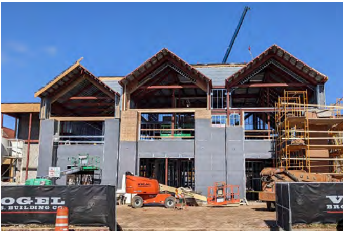
Full view of the structure of the library addition in late October
